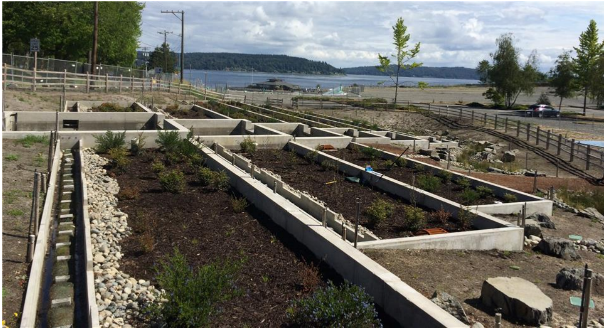
Figure 6: Photo of cascading rapid biofiltration treatment cells at the Point Defiance Stormwater Treatment Facility (Source: Contech Engineered Solutions)
