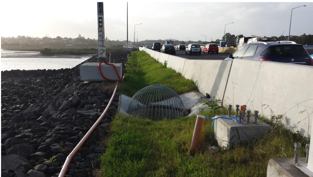
Figure 4: Photo of hybrid Swale & 'scruffy dome' entry Filtration device treatment train (Source: Causeway Alliance)
