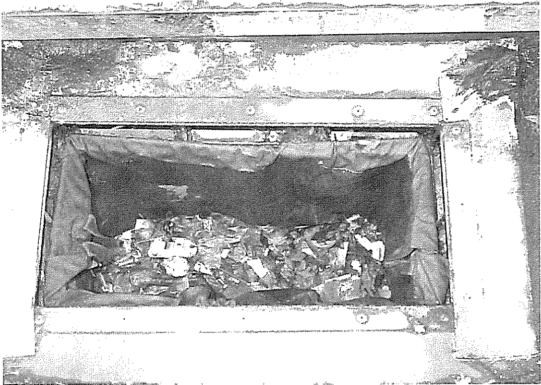
Photograph 2: The Enviropod Filter installed
